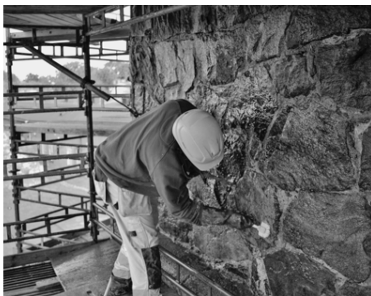
4.17) After grouting the mortar settles some hours before the wall is washed.
