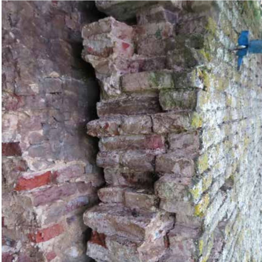
7.10) The cavity in the wall. On the left the core of the wall, dating from the 17th century. On the right the shell that was placed in front of it as a reparation in the 19th century. Between them the cavity of about 8 centimetres.
