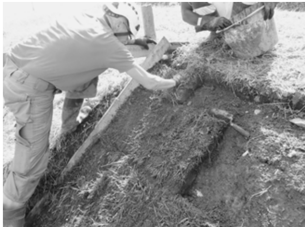
5.6) To have vegetation on the deep slopes it is easier with the grass tiles, Suomenlinna own transfer grass. Nowadays it is more difficult to find places where to get them because the places are recovering so slowly.
