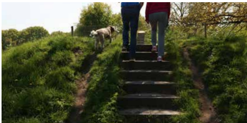
8.7) Stairs along the main path are highly vulnerable to vegetation erosion, leading to damage over time.
