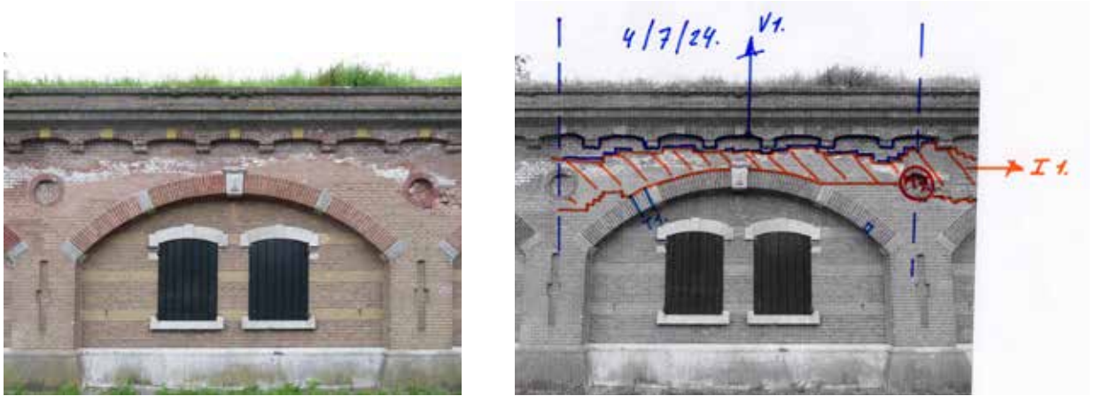
7.19) Picture showing the efflorescence in 2024. Next to it the same part of the wall with the proposed intervention marked on it. In blue the part where the cement joints need to be removed. In orange the part where the reparations of the previous restoration (in 2000) need to be taken out and replaced. As a test, part of this reparation will be taken out in October 2024 and replaced with new masonry. It will be tested in August 2025.
