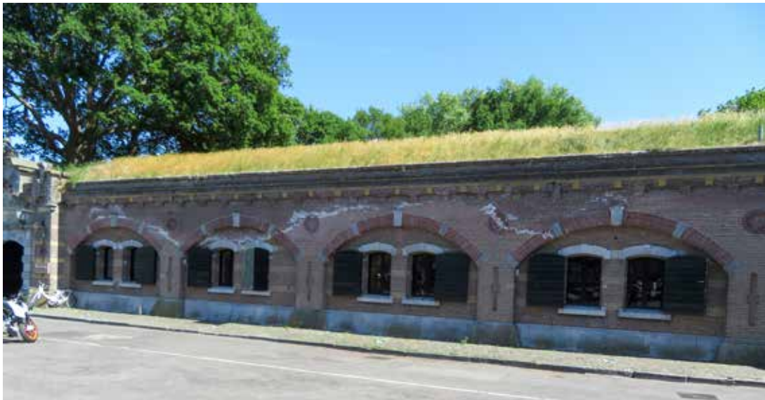
7.16) The façade of the Promers barracks, showing the salt efflorescence in 2019.
