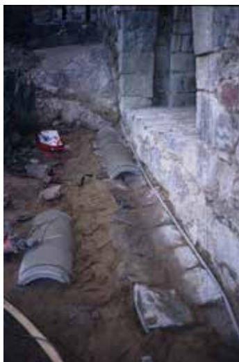
4.20-26) In the A13 shore work restoration project the principal objective besides wall repair was to prevent water getting into the structures, and if it did get in, to provide an exit for it. During the restoration project, the 18th-century drains and gutters were remade or repaired. Instead of using plastic drains with a short lifespan, the drains were built with stones and concrete pipes cut into two. Instead of using geotextile, the drains were covered gradually with cobble stones, uncrushed gravel, and sand. The gradually diminishing gravel is replacing the geotextile. This kind of infrastructure can easily be repaired in the future.
