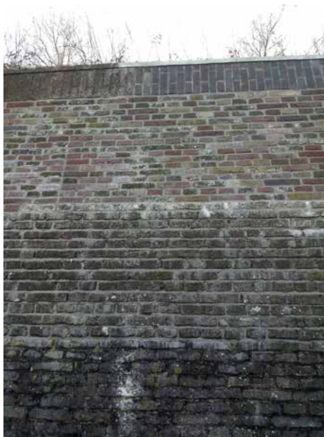
7.13) The efflorescence of lime that was visible on the wall in February 2019.
