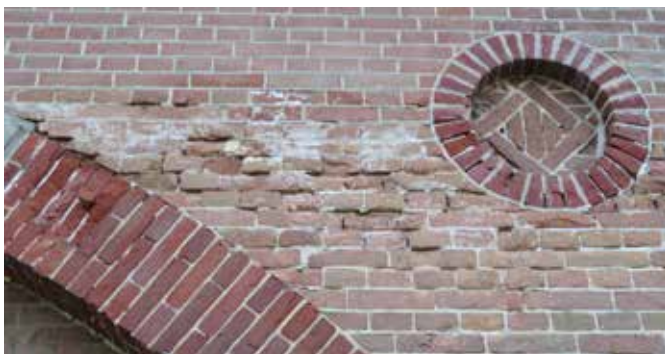
7.17) The damage caused by the salt in 2019.
