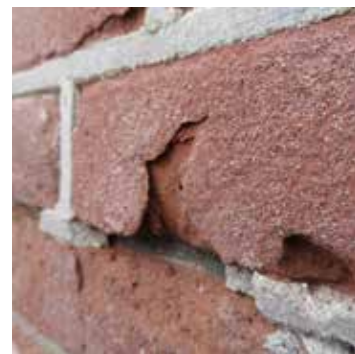
7.18) Detail of a splinter of brick about to come off in 2019. This is due to the salt crystallization in the masonry.
