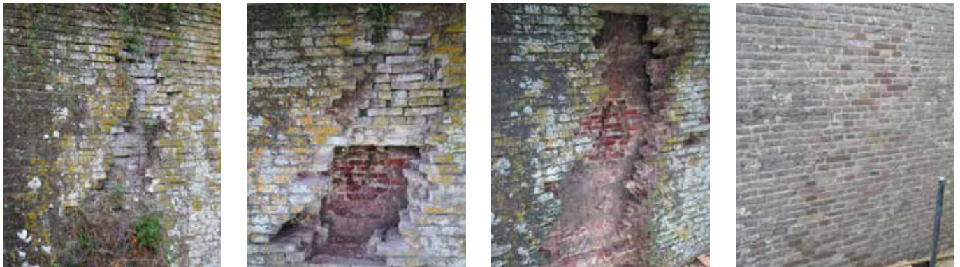
7.12) The restoration of a damaged part of the wall. From left to right:
