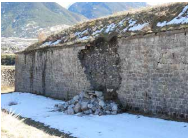
9.10) In winter 2018-2019, part of the wall of bastion 63 collapsed.
