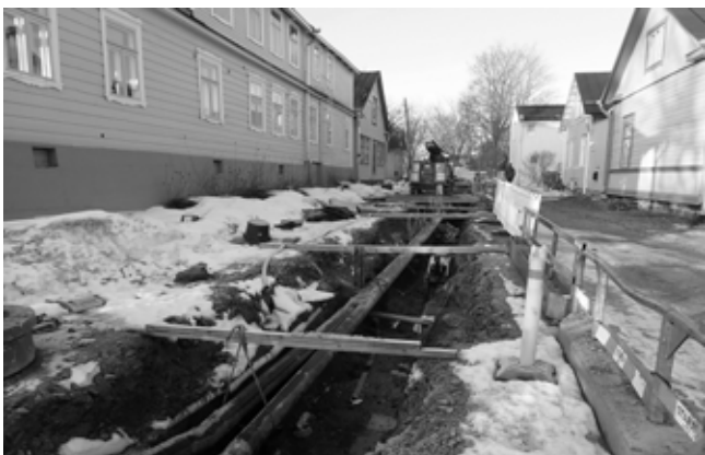
6.1) Typically, Suomenlinna's excavations are related to repair and restoration of buildings and landscape as well as infrastructure repair work.
