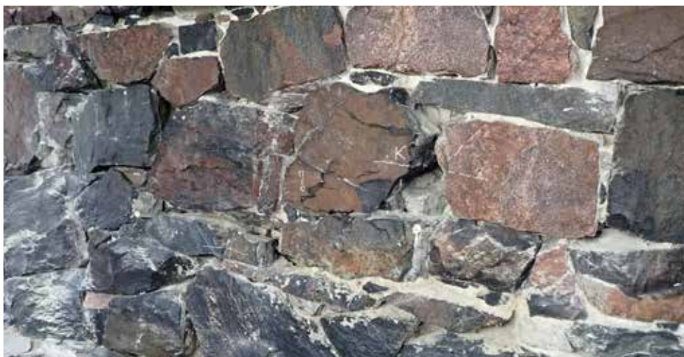
4.15) The first stage of wall repair is loosening pinning stones and extracting eroded mortar.
