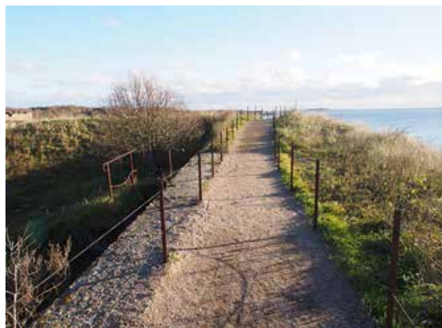
5.8) On the ramparts of Kustaanmiekka there has been build new path with modern structure and fences to avoid erosion.
