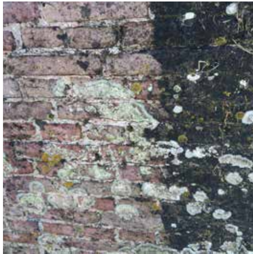
7.8) One of the things stated in the vision on the masonry was the preservation of lichen. On the right side, the wall with black algae and lichen. Damages and other irregularities are not visible without cleaning. On the left the wall after cautiously cleaning it with water at low pressure. The algae are removed, and the lichen stay.
