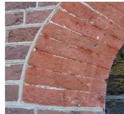
그림 172. 흐라블란트(Graveland)의 트롬펜뷰아흐(Trompenburgh) 성. 연마된 벽돌 사이의 줄눈은 최대한 얇게 만들고 붉은색을 칠해 줄눈을 완전히 덮었다. Fig. 172. Trompenburgh palace in 's Graveland. The joints between the polished bricks were made as thin as possible and were coloured red to completely cover up the joints.
