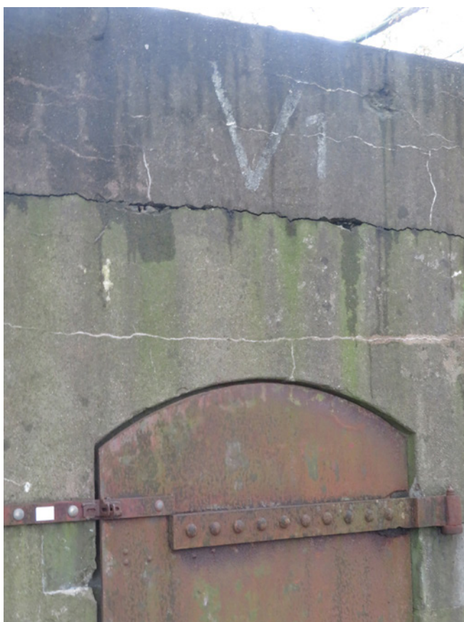
Figure 11. The horizontal cracking pattern on one of the shelters. The wide crack needs to be restored in the near future to prevent further damage (Authors).
